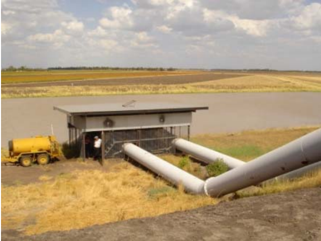
Irrigation Pump elevating runoff water (tail and storm) into the ring tank, picture taken from top of berm.
