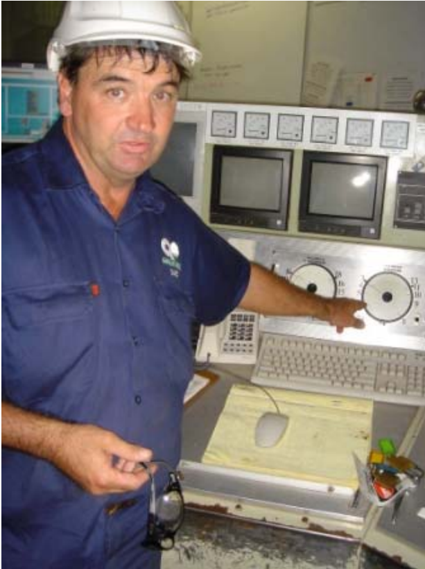
Cotton Gin General Manager showing how the control room controls the ginning process.
